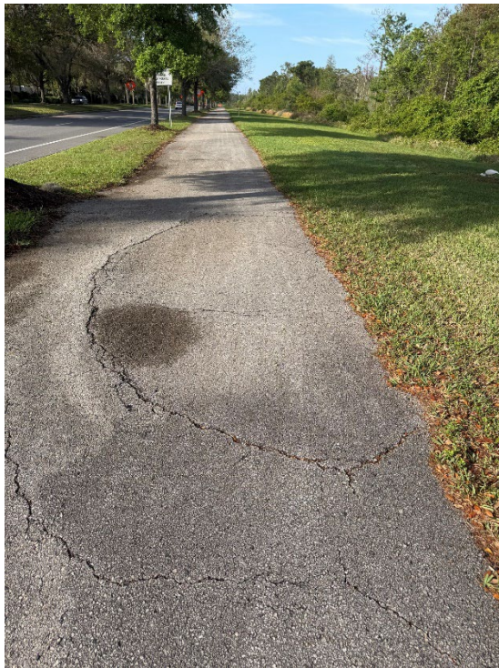
Photo 17.1 – Asphalt and Base Failure (New Photo – 2026 Assessment)
