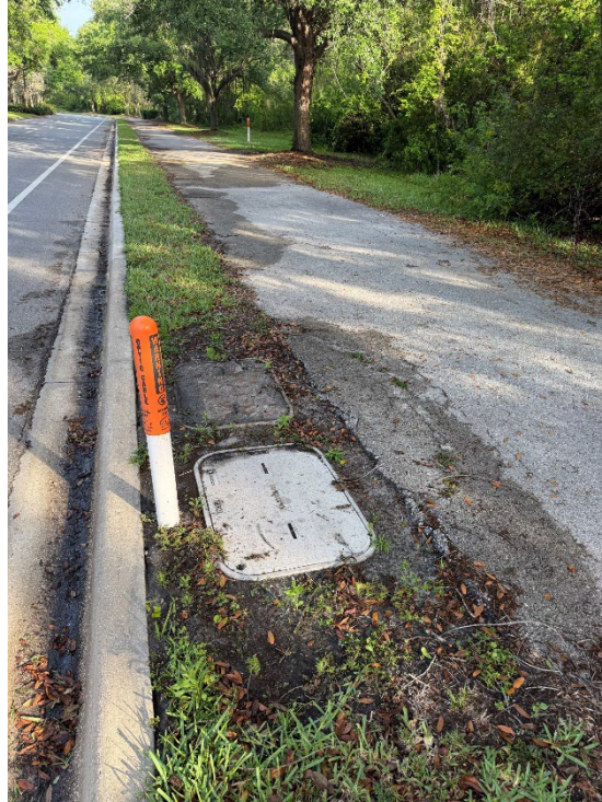
Photo 12 – Asphalt Raveling and Base Failure at Meter Box (No Observed Changes) (Refer to Prior Photo 16 - 2025 Assessment)
