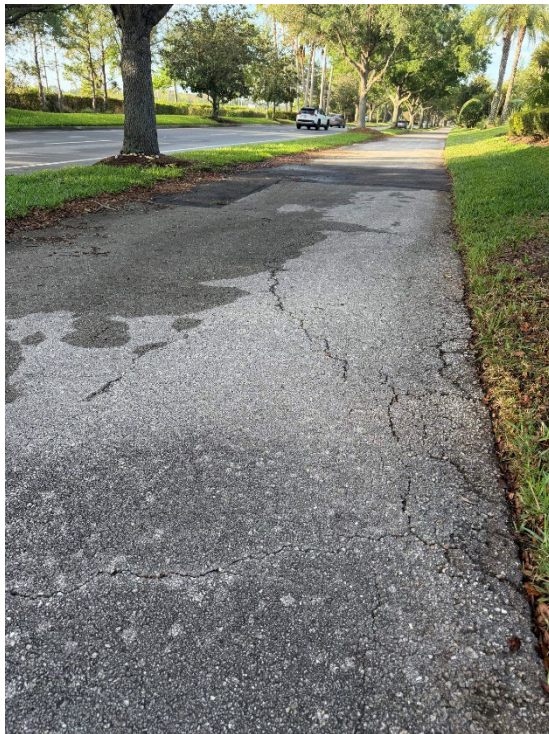
Photo 11 – Tree Roots Damaging Asphalt, Asphalt Failure (No Observed Changes) (Refer to Prior Photo 13 - 2025 Assessment)
