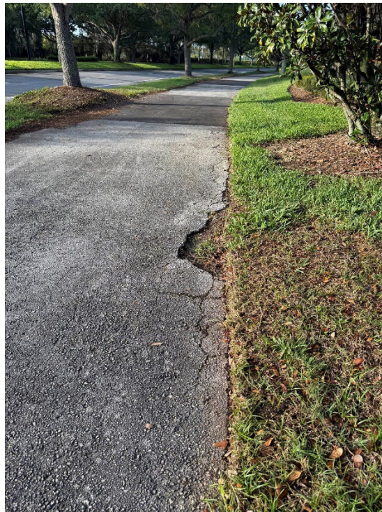
Photo 9.1 – Asphalt Raveling and Base Failure (New Photo – 2026 Assessment)
