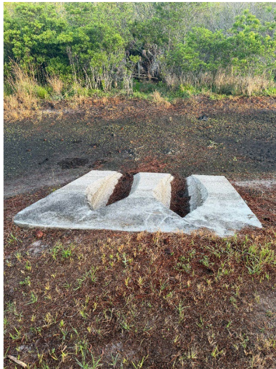
Photo 2 – Outfall into Spreader Swale in Good Condition (No Observed Changes) (Refer to Prior Photo 3 - 2025 Assessment)
