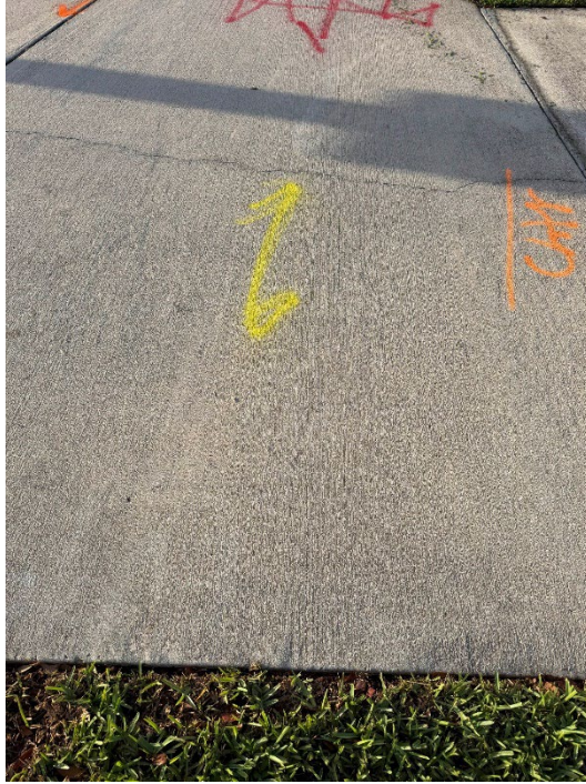
Photo 5 – Surficial Concrete Cracking Beginning of Pedestrian Path Lake Nona Blvd & Nemours Parkway (No Observed Changes) (Refer to Prior Photo 6 - 2025 Assessment)
