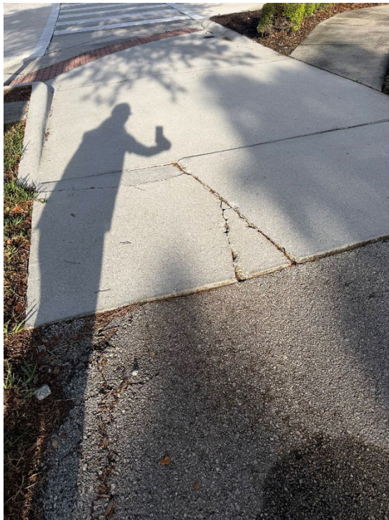
Photo 11.4 – Cracked Concrete on Sidewalk (New Photo – 2026 Assessment)
