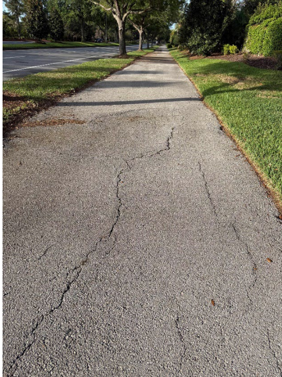
Photo 11.3 – Asphalt Cracking (New Photo – 2026 Assessment)
