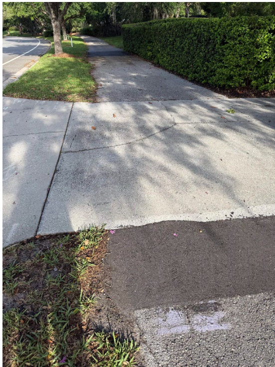
Photo 16 – Surficial Concrete Cracked in Driveway Apron (No Observed Changes) (Refer to Prior Photo 20 - 2025 Assessment)
