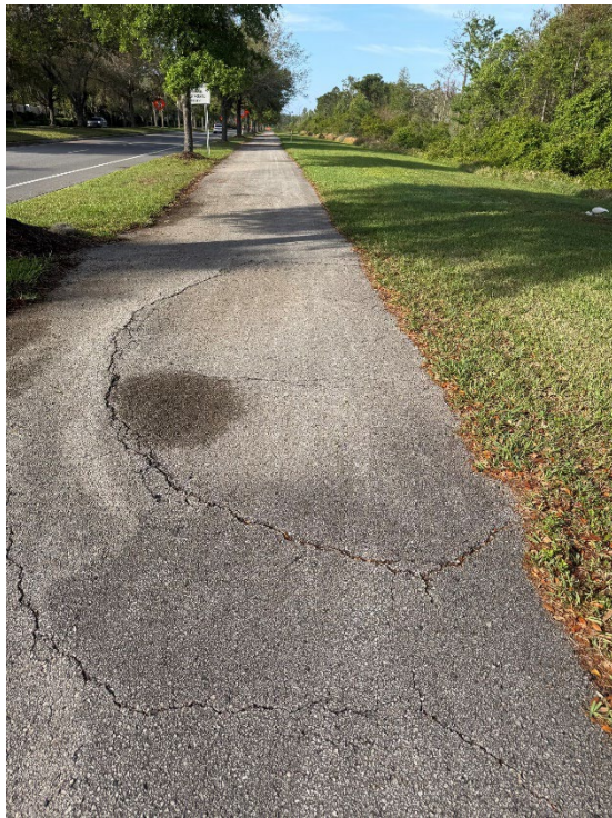
Photo 17.1 – Asphalt and Base Failure (New Photo – 2026 Assessment)
