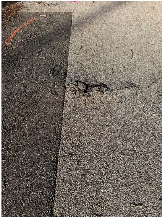
Photo 8 – Tree Roots Damaging Asphalt (No Observed Changes) (Refer to Prior Photo 10 - 2025 Assessment)
