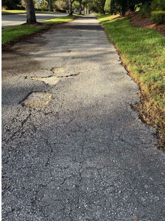
Photo 10 – Asphalt Damage (No Observed Changes) (Refer to Prior Photo 12 – 2025 Assessment)
