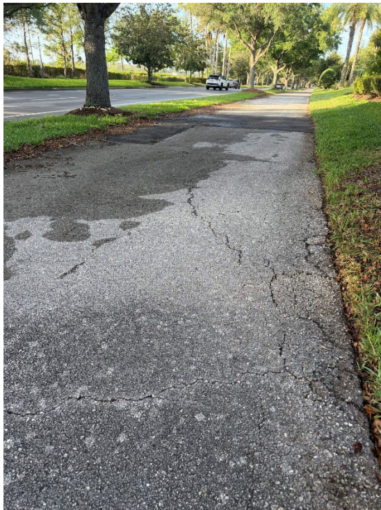
Photo 11 – Tree Roots Damaging Asphalt, Asphalt Failure (No Observed Changes) (Refer to Prior Photo 13 - 2025 Assessment)
