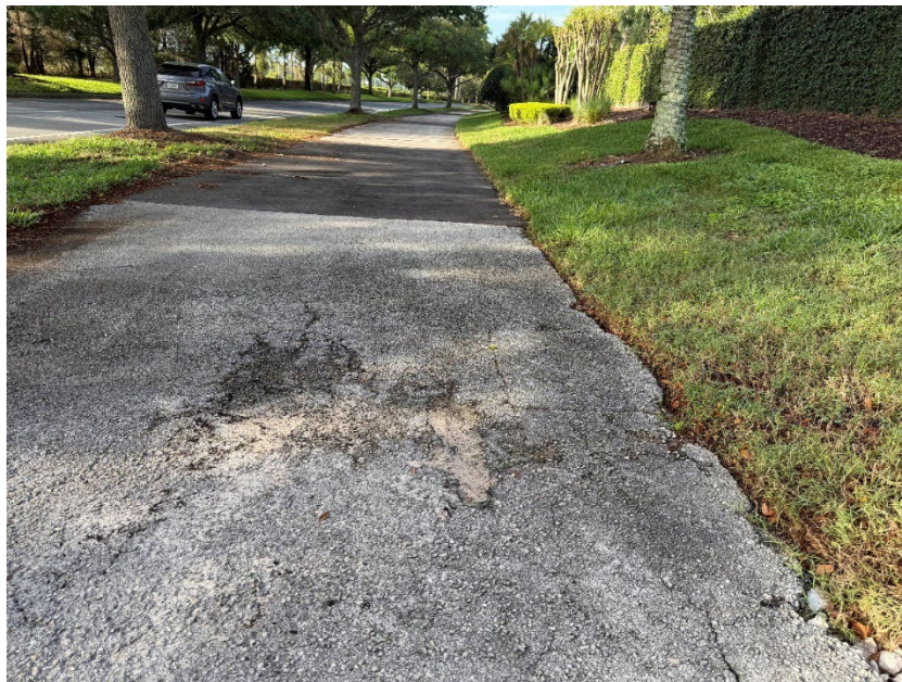
Photo 11.2 – Additional Asphalt Damage and Base Failure (New Photo – 2026 Assessment)
