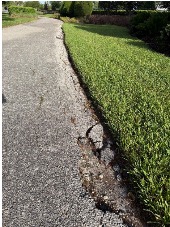
Photo 14.1 – Asphalt Raveling and Base Failure (New Photo – 2026 Assessment)
