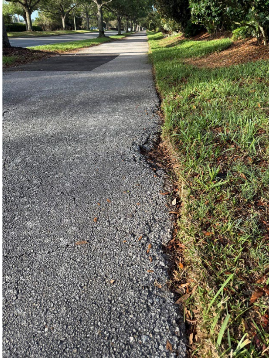
Photo 11.1 – Typical Asphalt Raveling and Failure (New Photo – 2026 Assessment)
