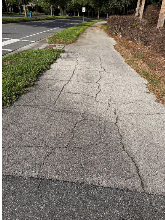
Photo 17 – Alligator Cracking (No Observed Changes) (Refer to Prior Photo 21 - 2025 Assessment)
