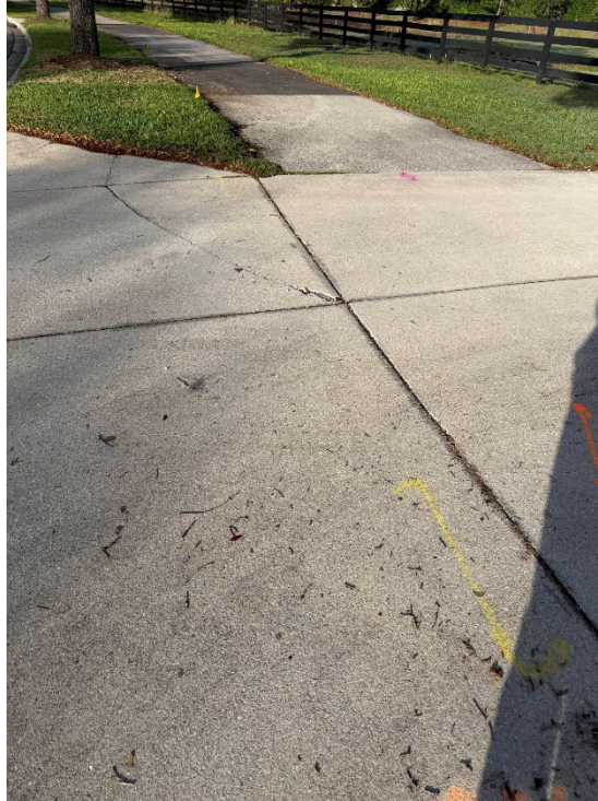
Photo 9 – Surficial Concrete Cracks at Construction Entrance (No Observed Changes) (Refer to Prior Photo 11 - 2025 Assessment)
