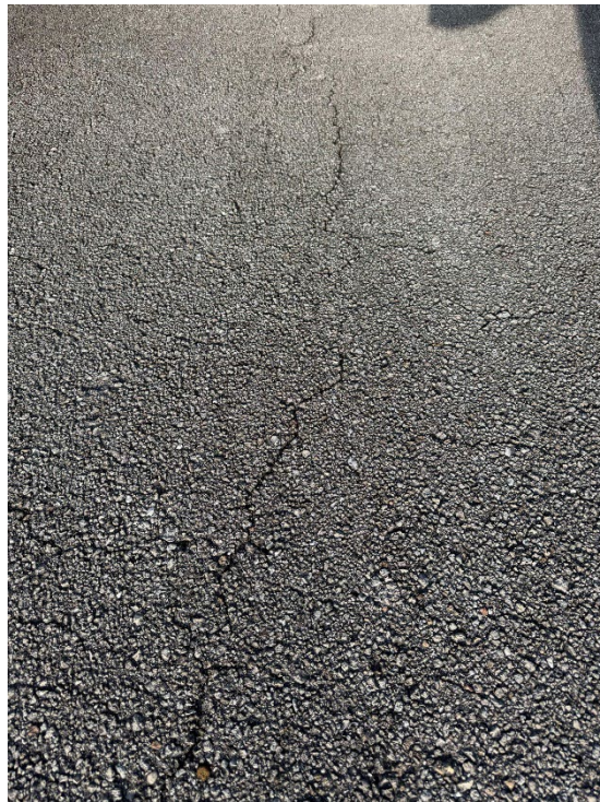
Photo 7 – Typical Asphalt Raveling (No Observed Changes) (Refer to Prior Photos 8 and 9– 2025 Assessment)
