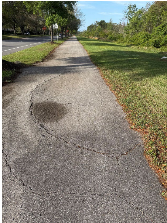
Photo 17.1 – Asphalt and Base Failure (New Photo – 2026 Assessment)
