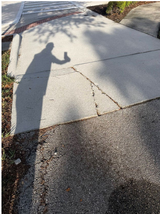
Photo 11.4 – Cracked Concrete on Sidewalk (New Photo – 2026 Assessment)
