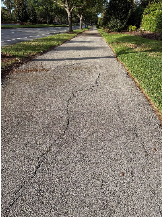
Photo 11.3 – Asphalt Cracking (New Photo – 2026 Assessment)
