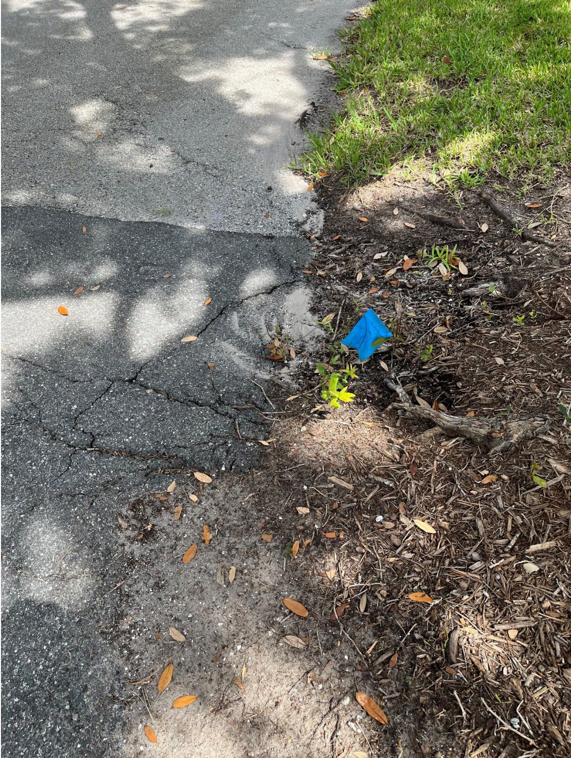
Photo 14 – Poor Quality Asphalt Patch
