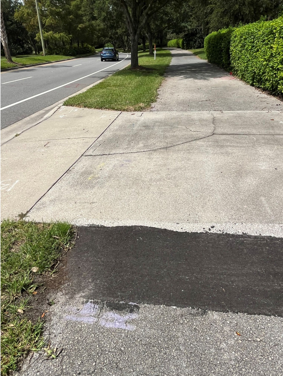
Photo 20 – Surficial Concrete Cracks in Driveway Apron
