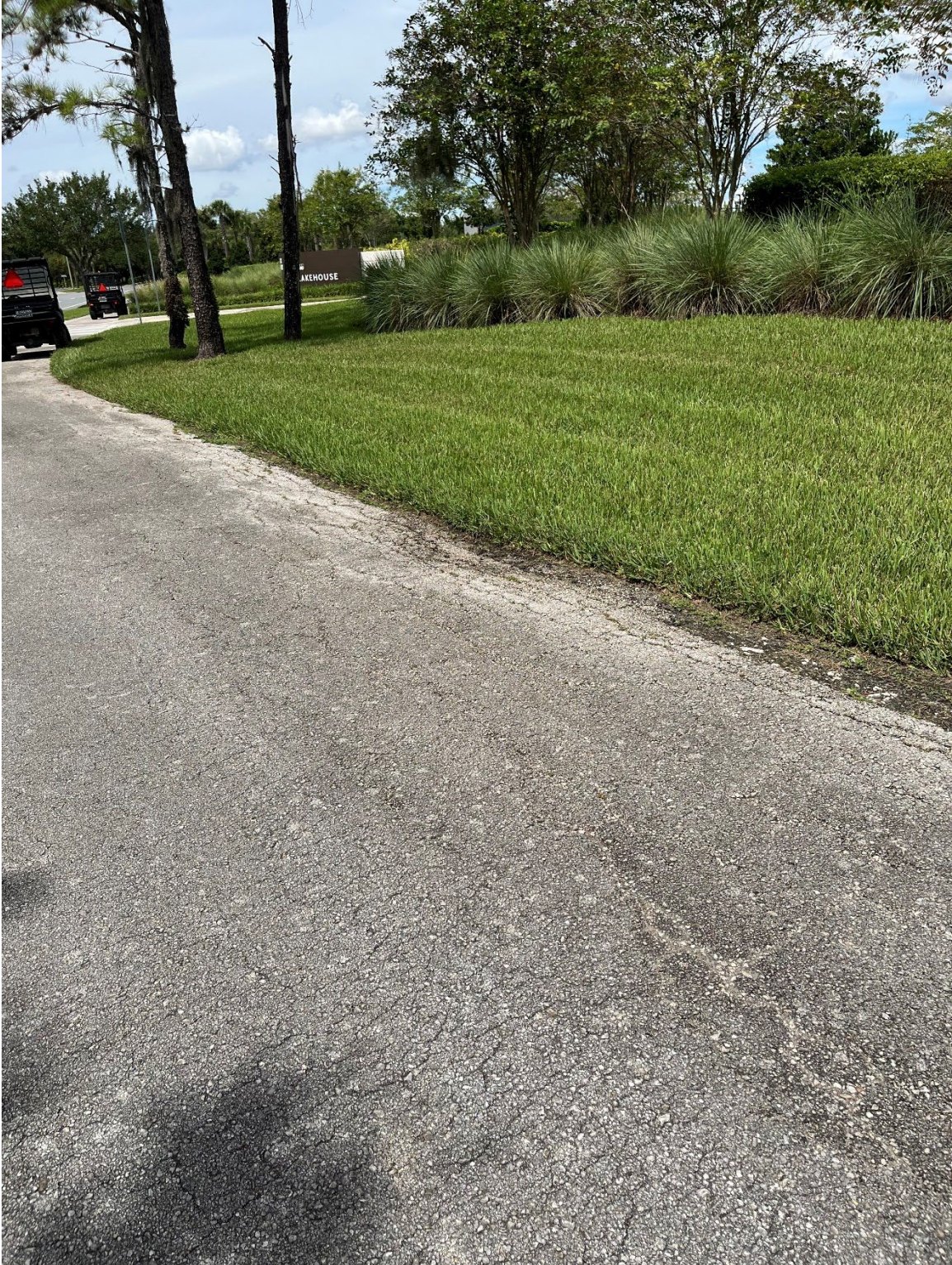
Photo 19 – Asphalt Raveling and Base Failure
