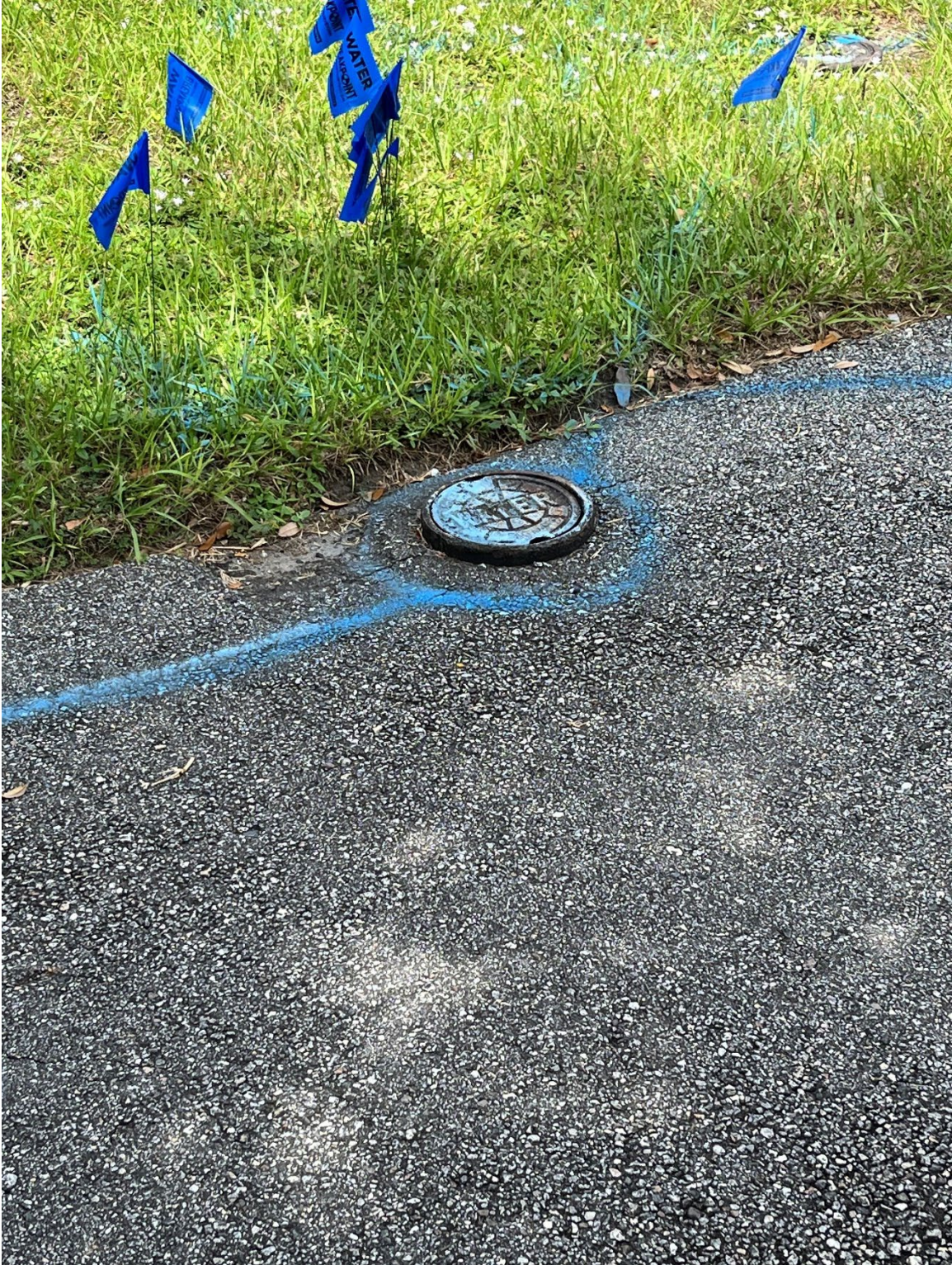
Photo 26 – Valve Cover Reveal Approximately 1 inch
