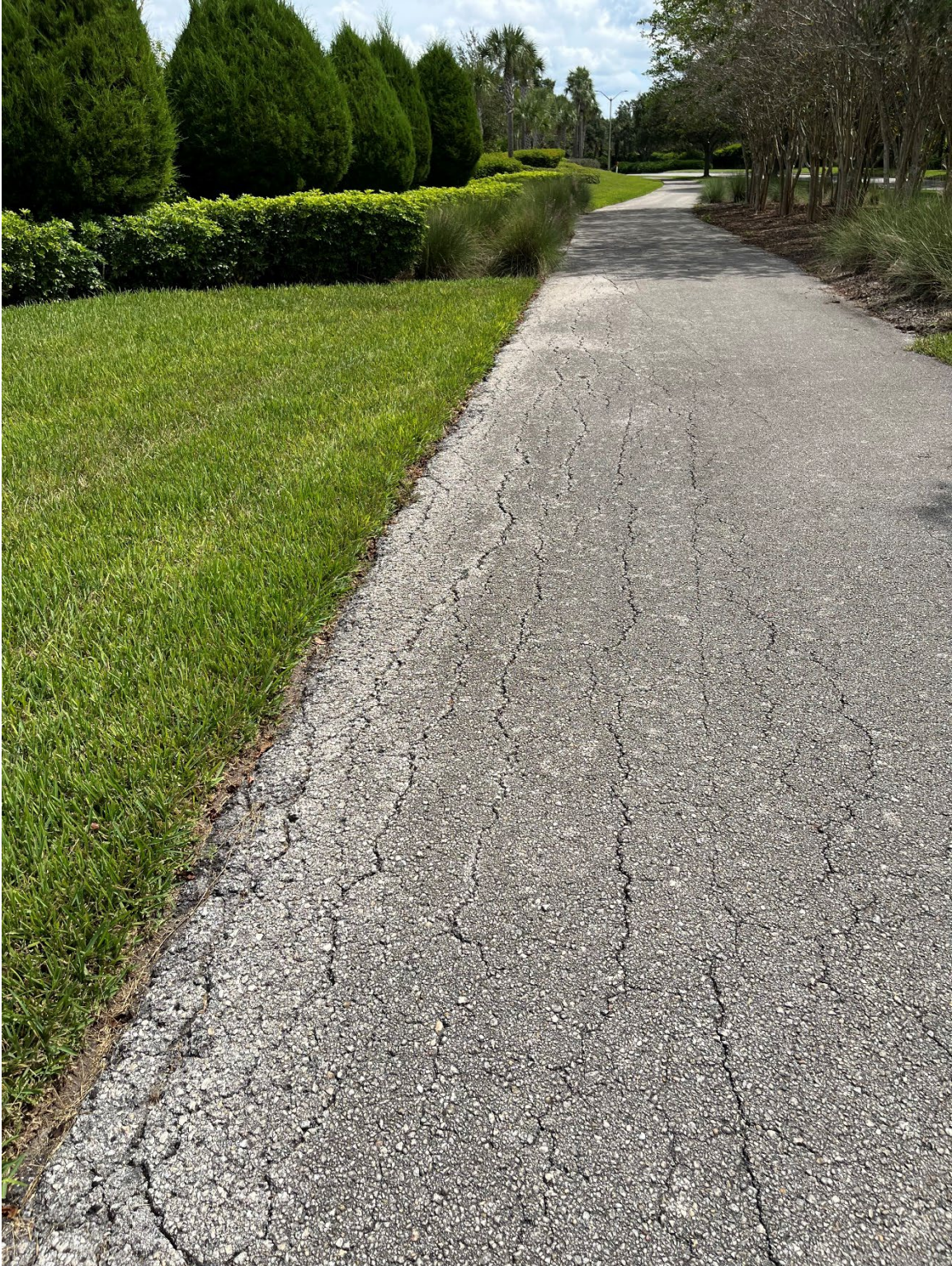
Photo 17 - Asphalt Raveling and Base Failure
