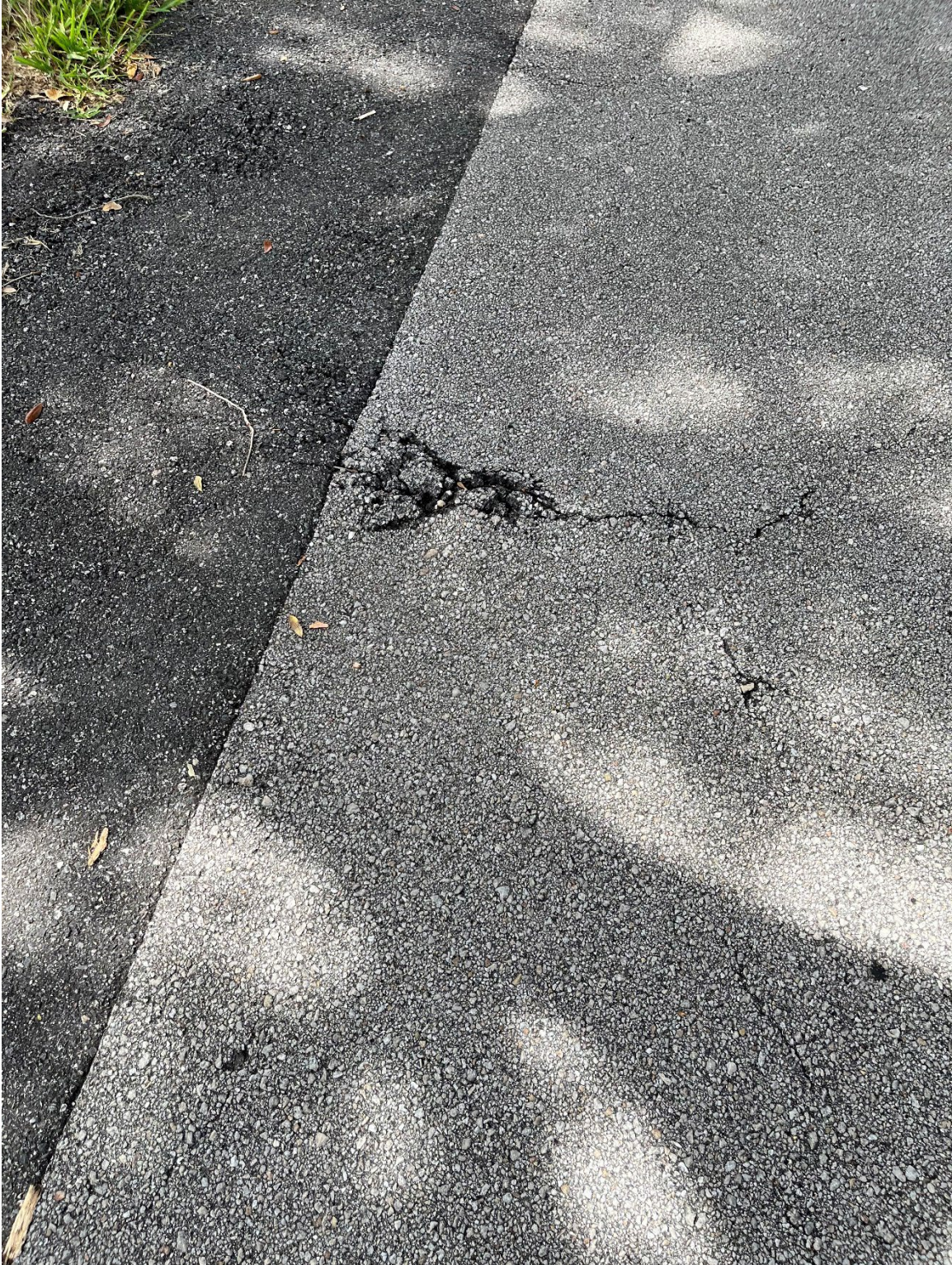
Photo 10 – Tree Roots Damaging Asphalt
