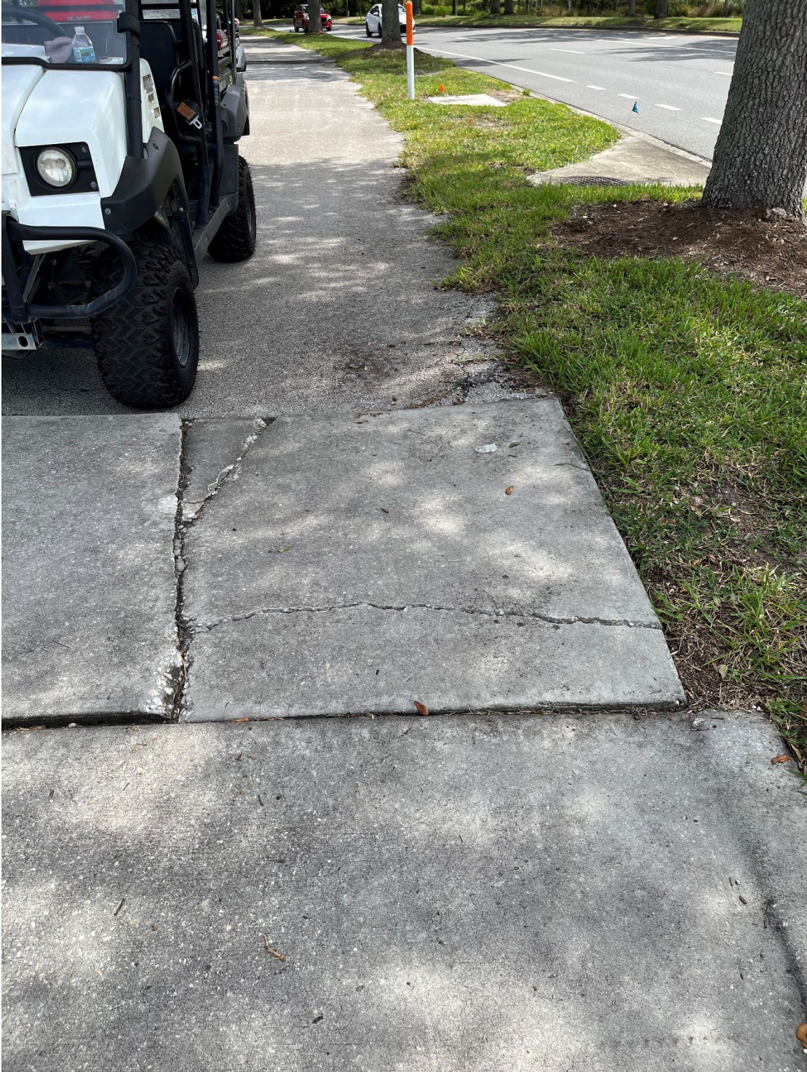
Photo 15 – Tree Roots Damaging Concrete
