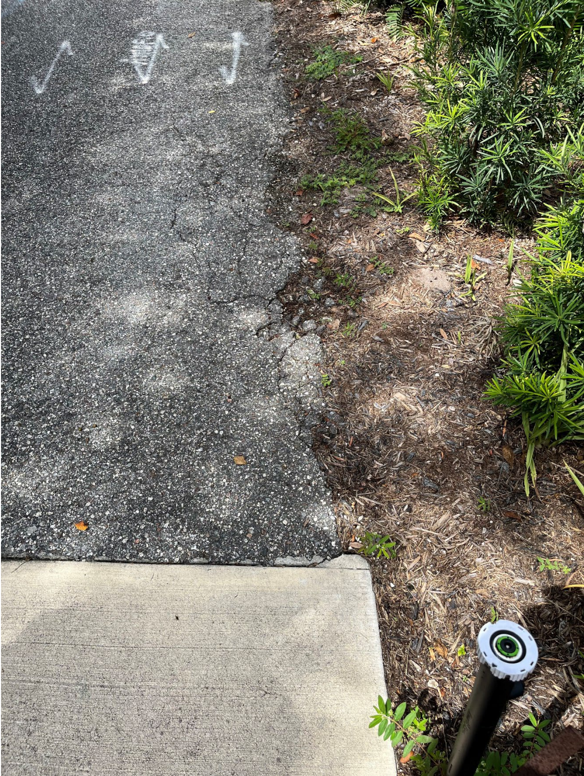
Photo 7 – Asphalt Raveling and Base Failure
