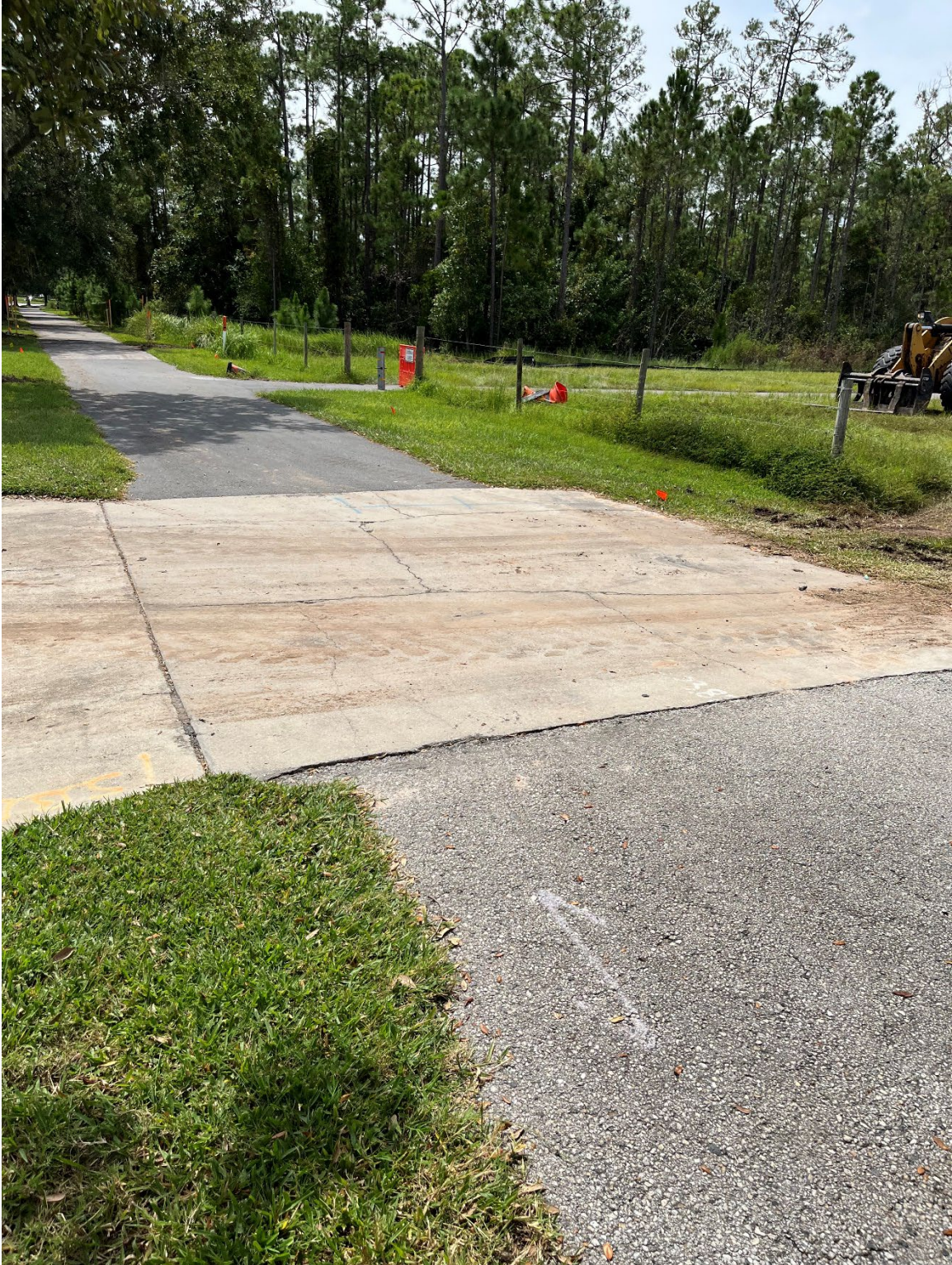
Photo 22 – Surficial Concrete Cracks in Driveway Apron
