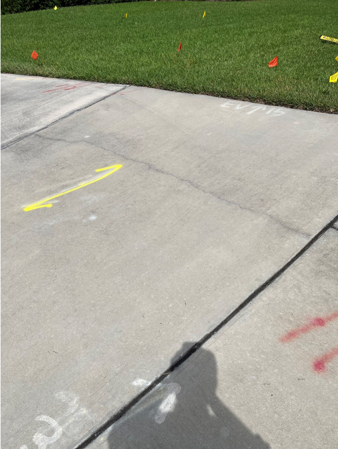
Photo 6 – Surficial Concrete Cracking Beginning of Pedestrian Path (Lake Nona Blvd and Nemours Parkway)
