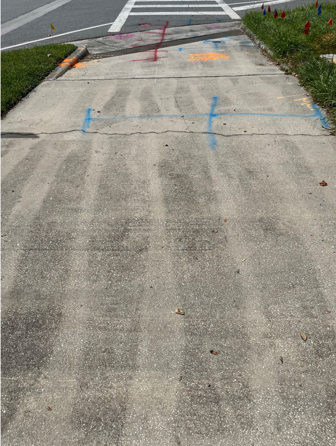
Photo 25 – Surficial Concrete Cracks
