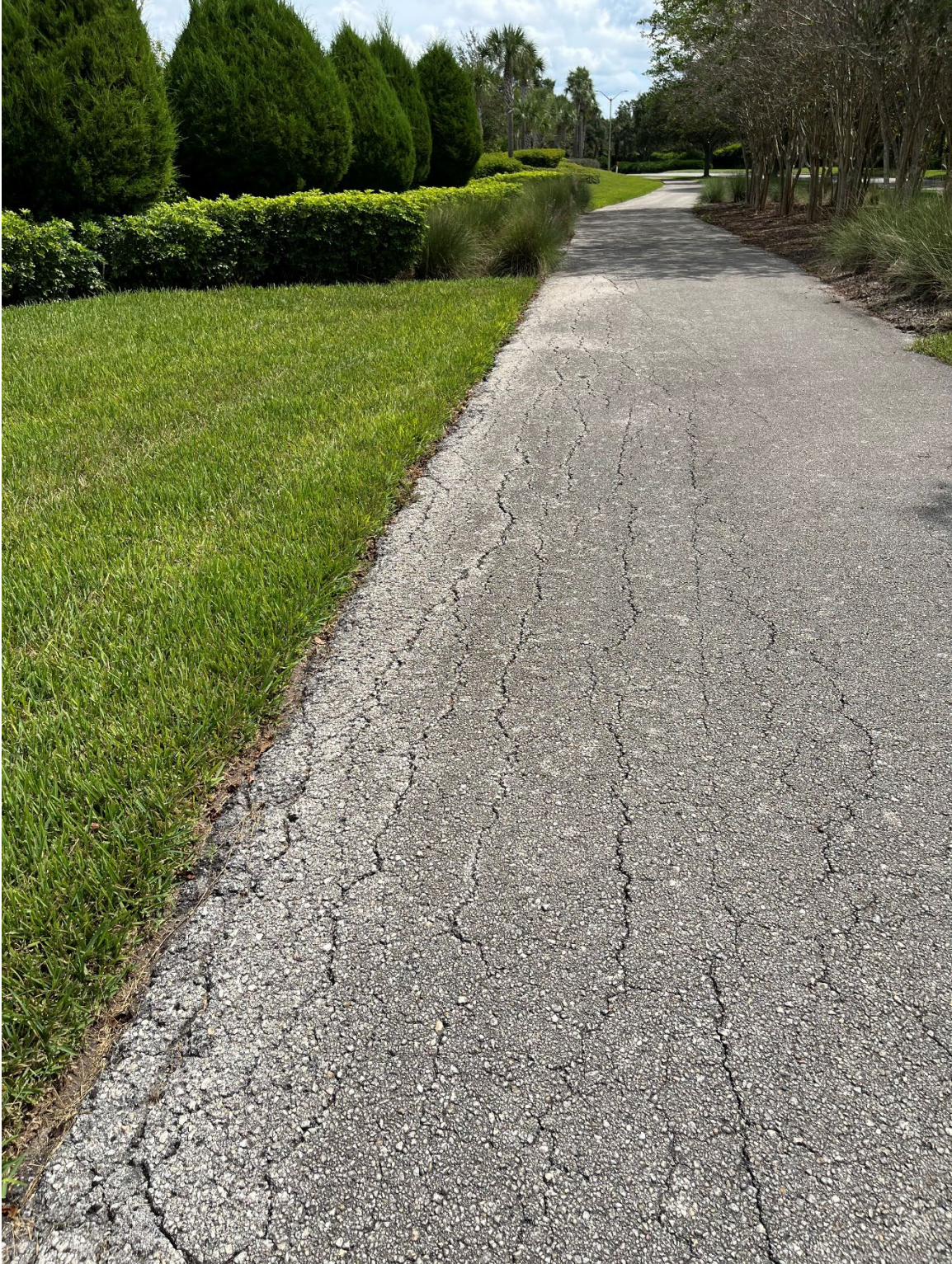
Photo 17 - Asphalt Raveling and Base Failure
