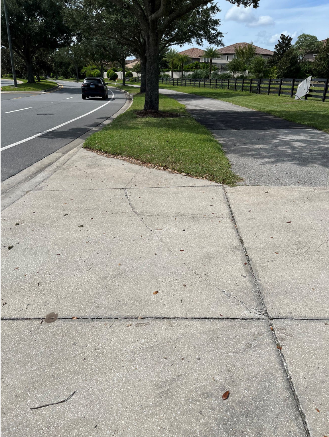
Photo 11 – Surficial Concrete Cracks in Driveway Apron
