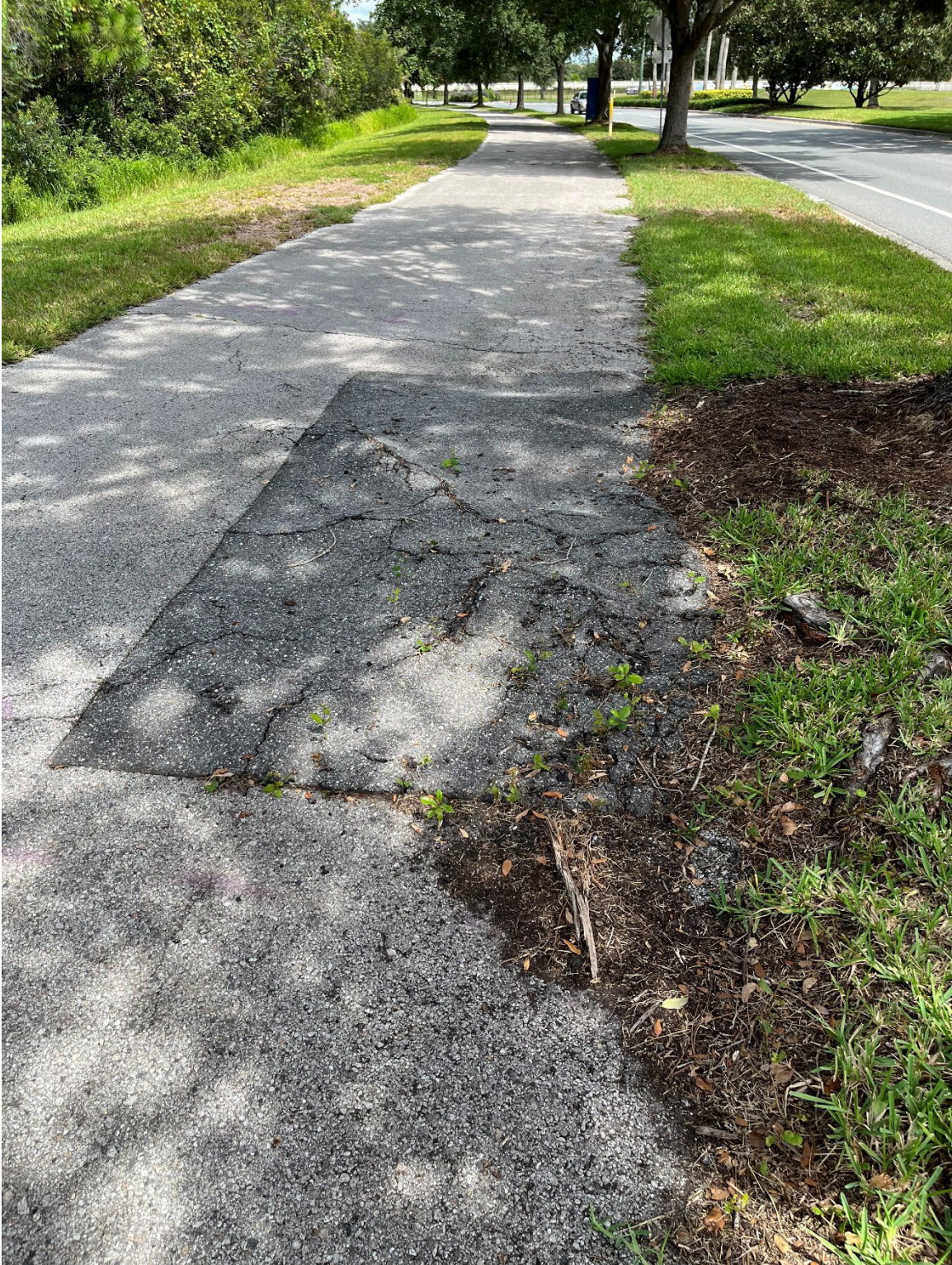
Photo 24 – Tree Roots Damaging Asphalt
