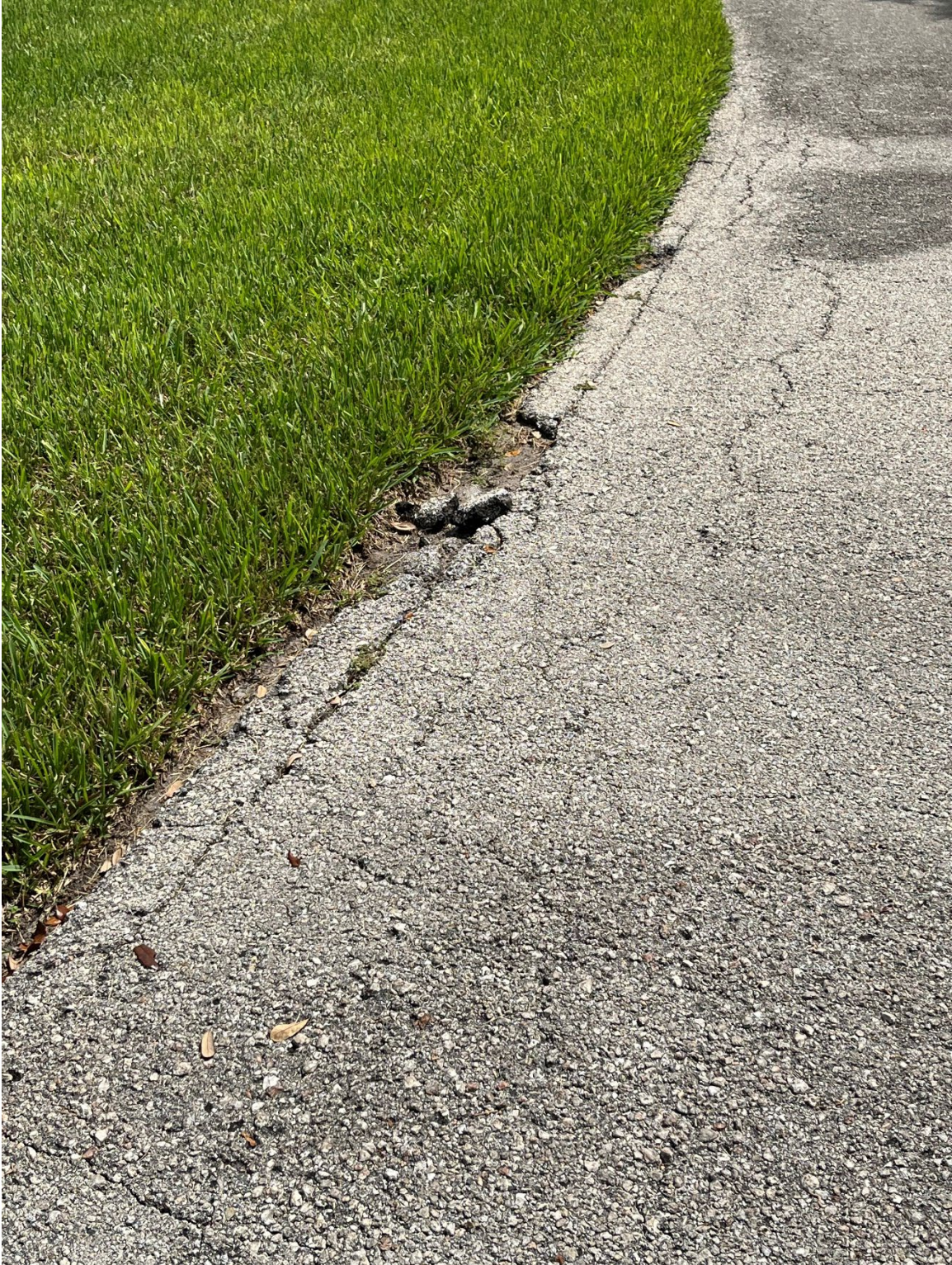
Photo 18 – Asphalt Raveling and Base Failure
