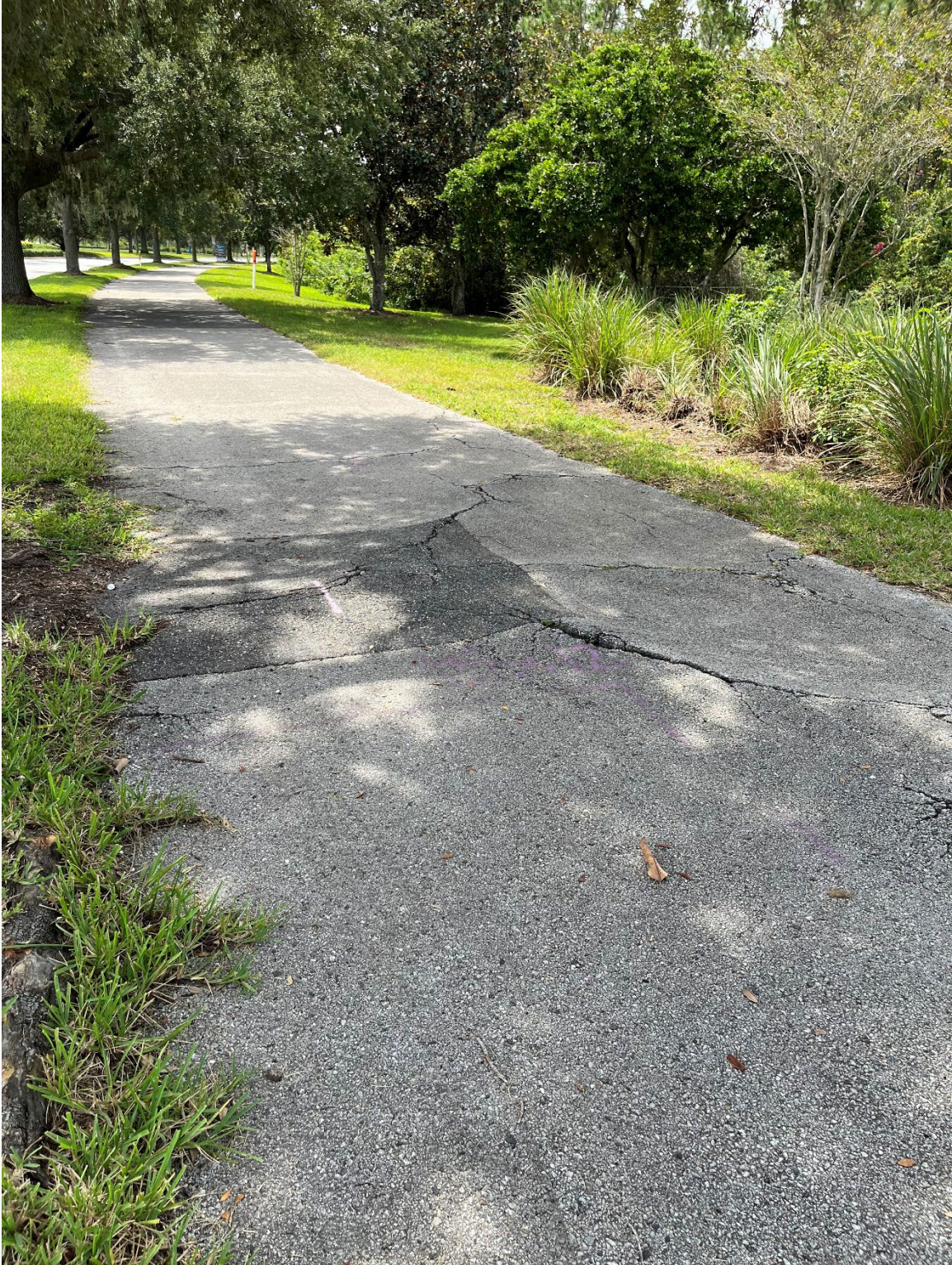
Photo 23 – Tree Roots Damaging Asphalt
