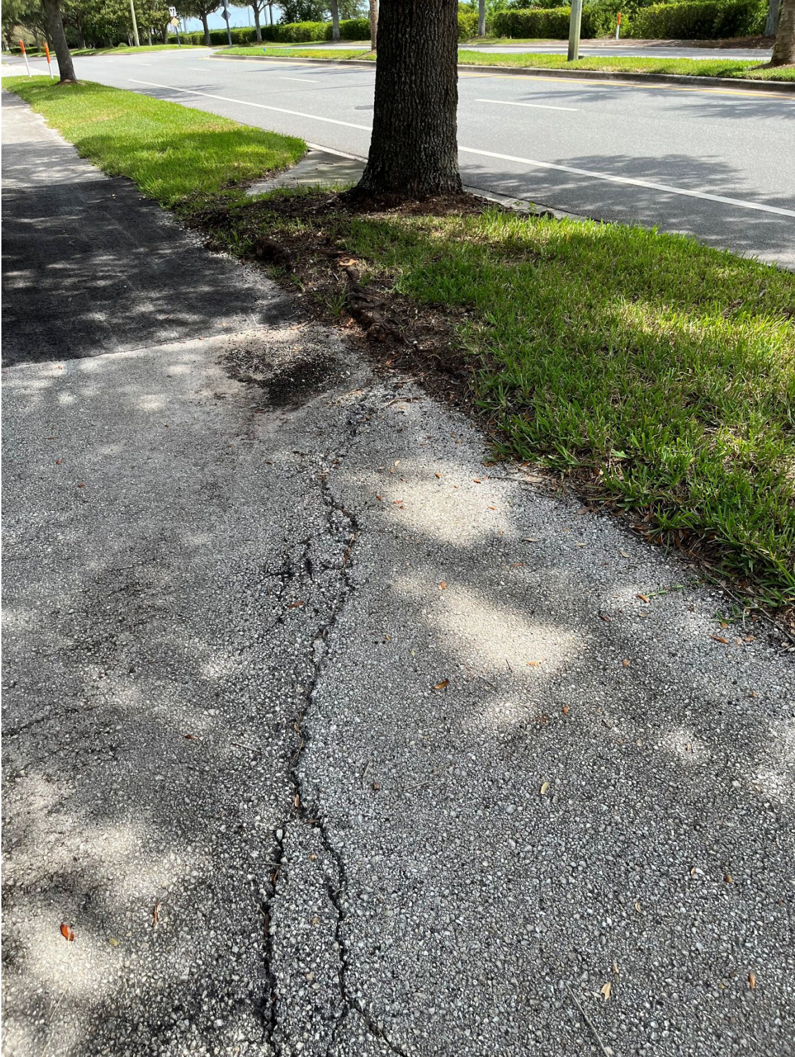
Photo 13 – Tree Roots Damaging Asphalt
