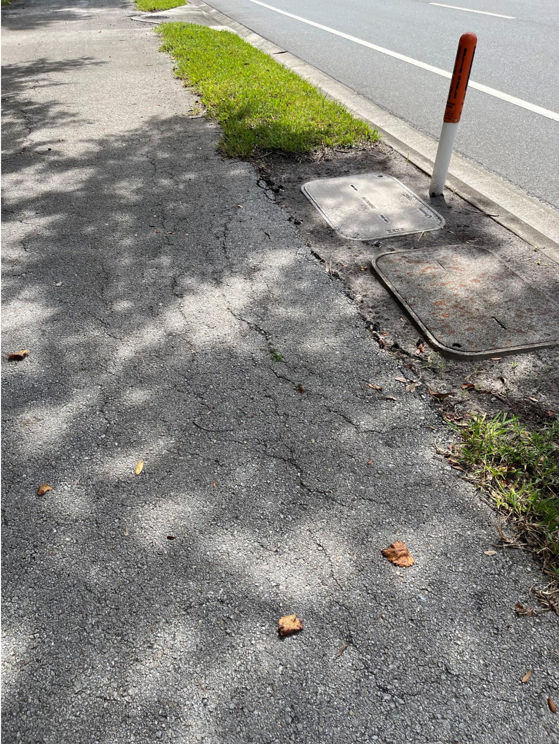
Photo 16 – Asphalt Raveling and Base Failure at Meter Box
